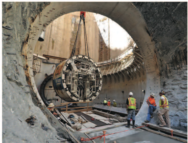
Fig. 4 Charismatic boring machine used to dig tunnel below Anacostia River. Image courtesy of DC Water.
